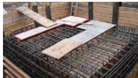
The overflow chamber in progress: the walls are seven metres high and 16 inches thick.
